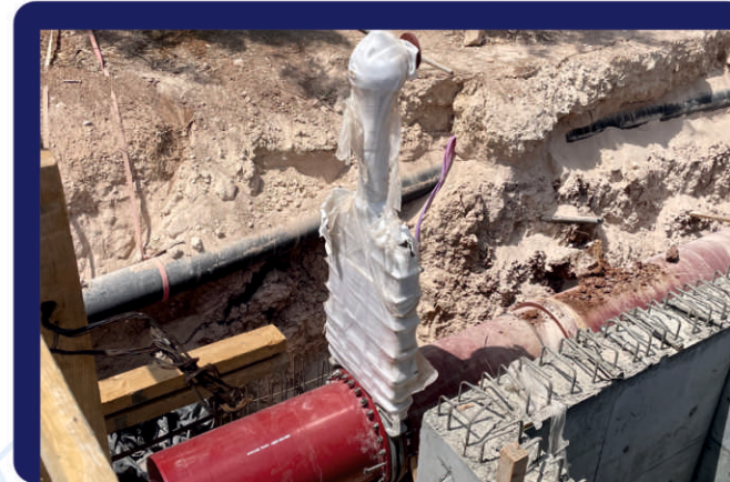
1000MM (40") WASTE WATER TREATMENT PLANT, RAMATHA, MIDDLE EAST
