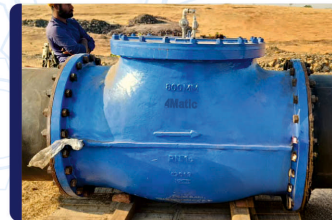
800MM (32") WATER TREATMENT PLANT, EGAT THAILAND
